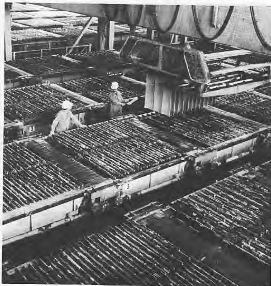
FIGURE 24.31 Electrolytic Cells at Copper Pass
