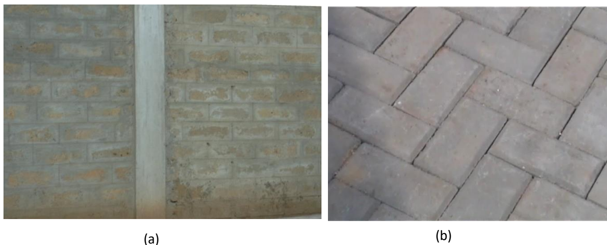
Fig. 4.15 (a) concrete bricks and pillars for strong wall and (b) concrete pavers
