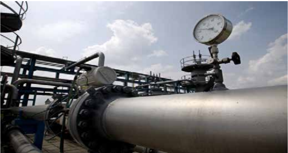
Figure 2.2.7: Showing oil pipeline in Nigeria
