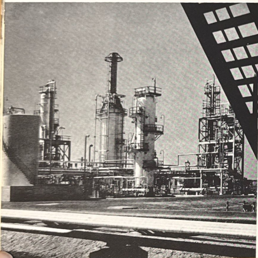
The lube plant, as it is called by the refiners, has a capacity of 900 barrels a day and produces 104 types of lubricating oils.
